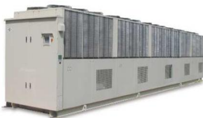
AIR COOLED CHILLER (5CS)
